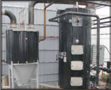
Boiler with the Waste Heat Boiler
